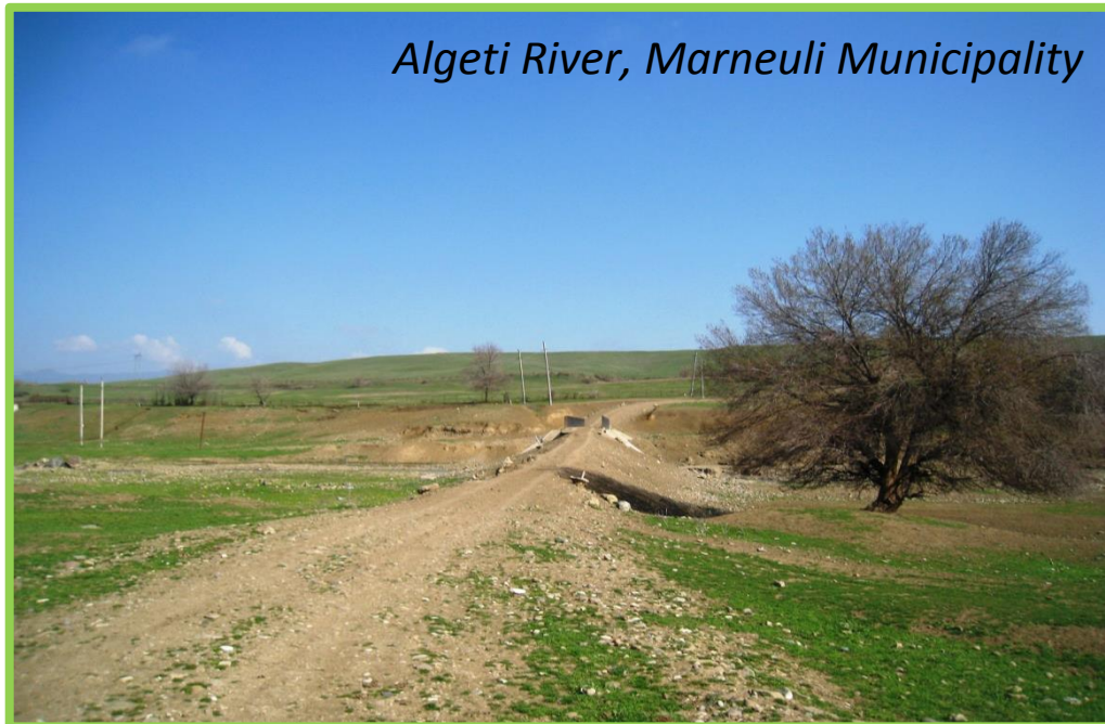
Access Road & Bridge approach needs up grading
