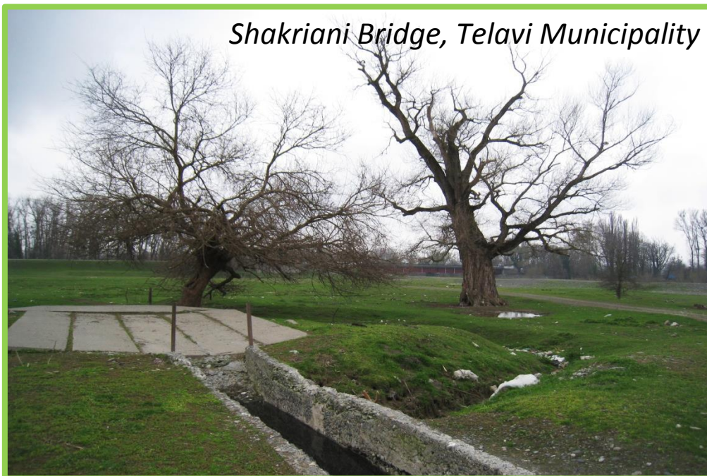
Old Dip needs up grading
